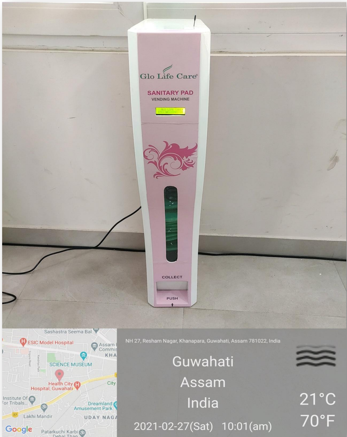
Sanitary Pad Vending Machine installed at KKHSOU, Khanapara, Guwahati-22
